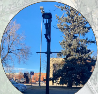
Holophane pedestrian pole installation.
